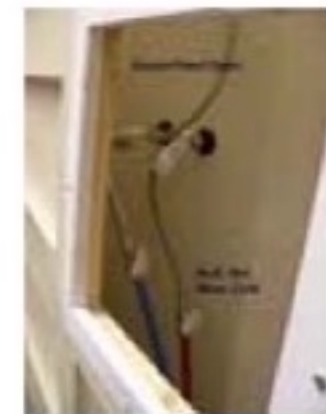
Side Access Panel Plumbing
